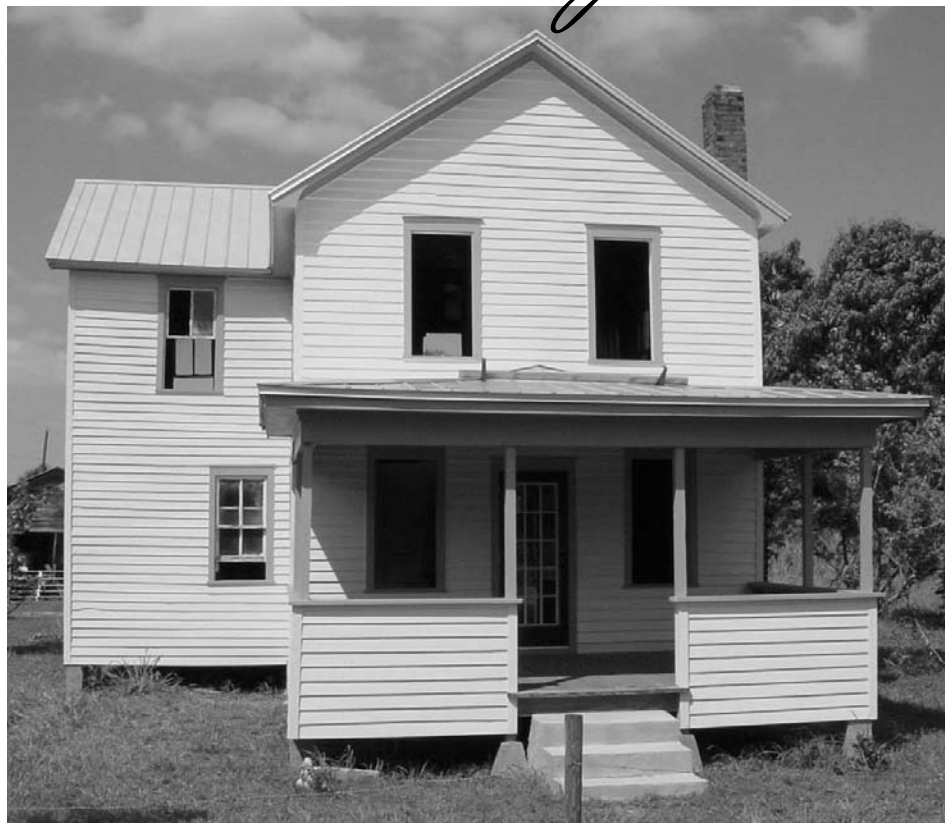
With fresh paint and a new roof, in March 2004 the Flint Home is undergoing window restoration.
